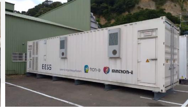
Energy Storage System
