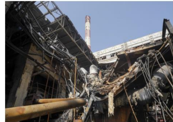
A damaged thermal power plant near Kharkiv, Ukraine, on April 12. Photographer: Andrii Marienko/AP Photo
